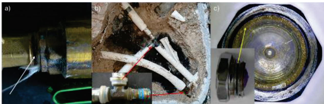
Figure 1: Failed brass components from building A (a), B (b), and C (c). The white arrow in (a) indicates the fracture of the outside thread; red arrows in (b) show the position of T-fittings inserted in the cement screed on the floor; and the yellow arrow in (c) indicates the position of the fracture at the outer thread of the plug.
