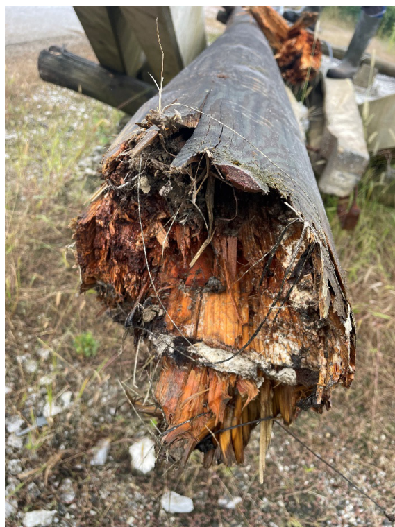
Fig. 3: Degraded utility poles in the storage yard
