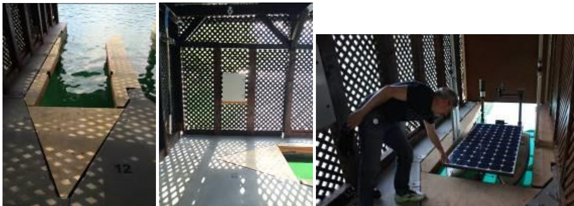
Figure 18: Installation of the service wharf at boat house of Vila Bled (timber elements with electricity).
