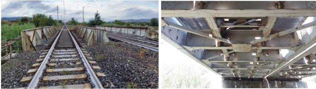
Figure 1. View from the top (left) and bottom (right) of the old steel riveted bridge.
