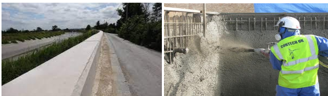
Figure 21: An example of using the fibre reinforced concrete for construction of a flood wall (left), from ADFIL (2015), and its application by the sprayed concrete technology (right), from Contech UK, (2022).
