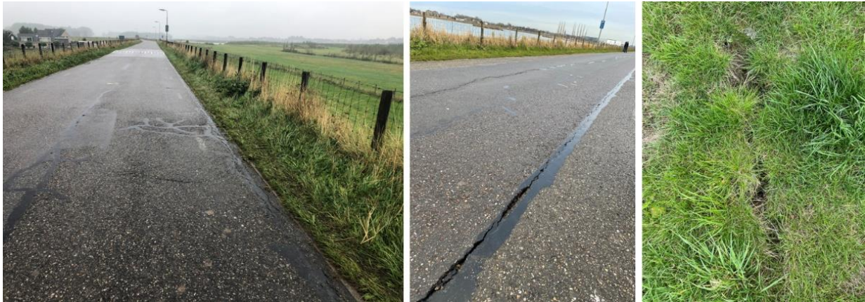
Figure 10: Cracks on the Oostmolendijk crest road and on the embankment slopes, from Kovačević et al. (2022)
