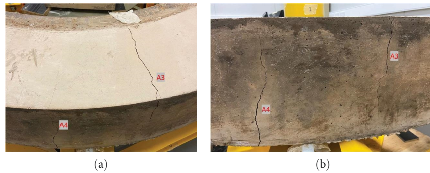
FIGURE 11: Crack A3 (occurred on day 22) and Crack A4 (occurred on day 39): (a) isometric view and (b) side view.
