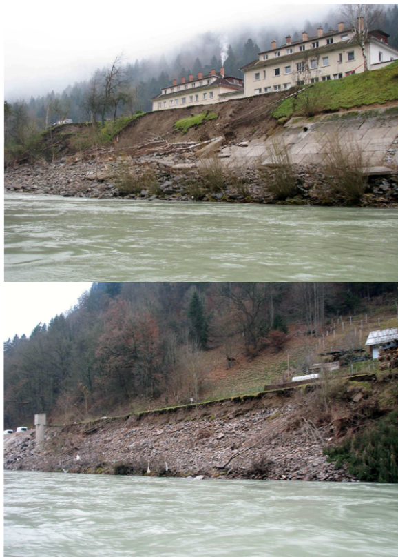
Fig. 9. Some examples of damaged banks of reservoirs on the Drava River after extensive floods (Photos: A. Geršak).
