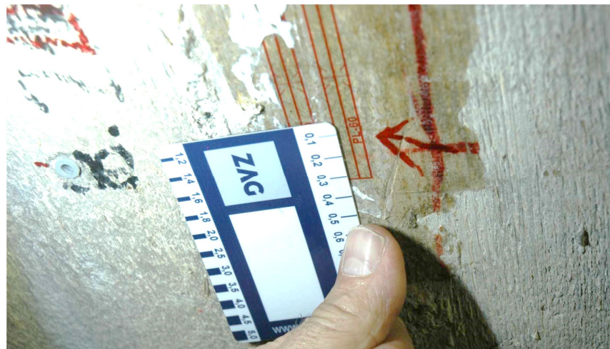
Figure 23. 0.1 mm wide crack under the strain gauge SG8.
