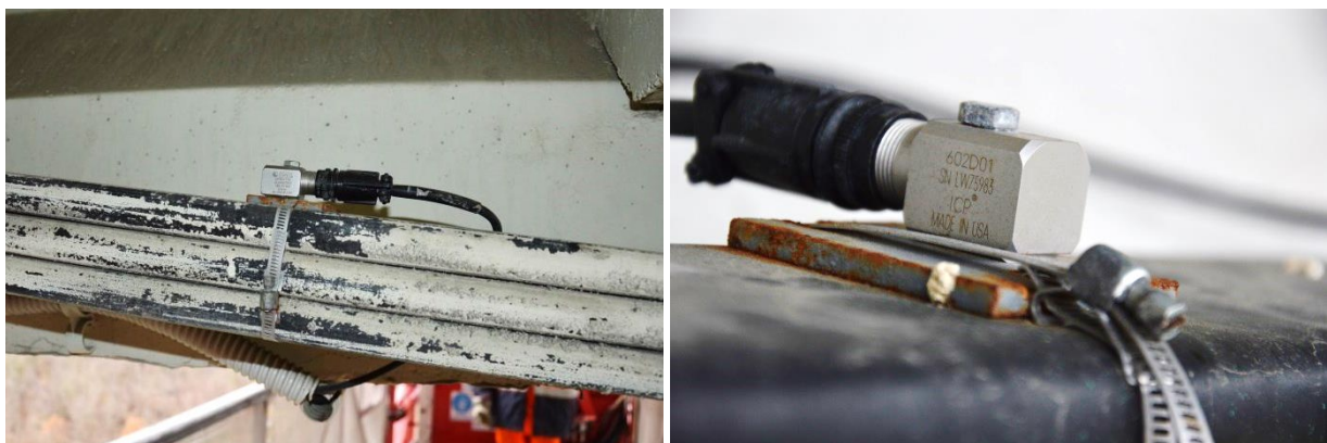
Figure 8: Prestressing cable consisting of 3 HDPE tubes and overall 6 strands with accelerometer (left) and accelerometer (right) on the left viaduct
