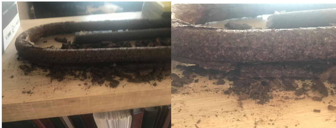
Figure 7. Reduction of armature cross-section caused by corrosion from direct contact with the external environment.
