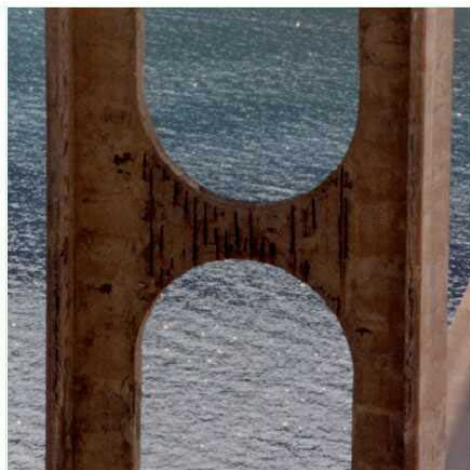
Figure 4. a) cracks on the pillar in 1993.;
