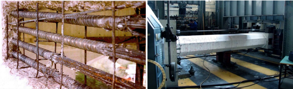
Figure 3: Corrosion of prestressed I-shaped beam in 1996 (left) [6] and experimental studies of scaled bridge pier (right)
