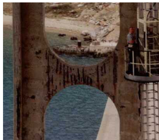
b) loosening of the flange edges and widening of the cracks 2001.
