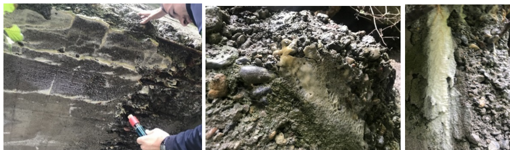
Figure 3: Degradation concrete elements
