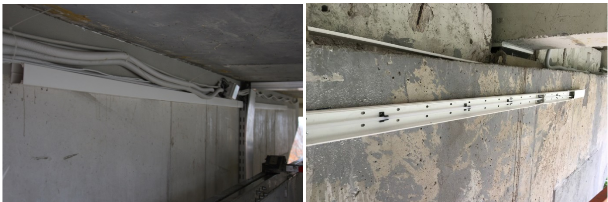
Figure 12: Smartec SOFO sensor, installed at the side of the pier cap on the left viaduct: covered (a) and uncovered (b)
