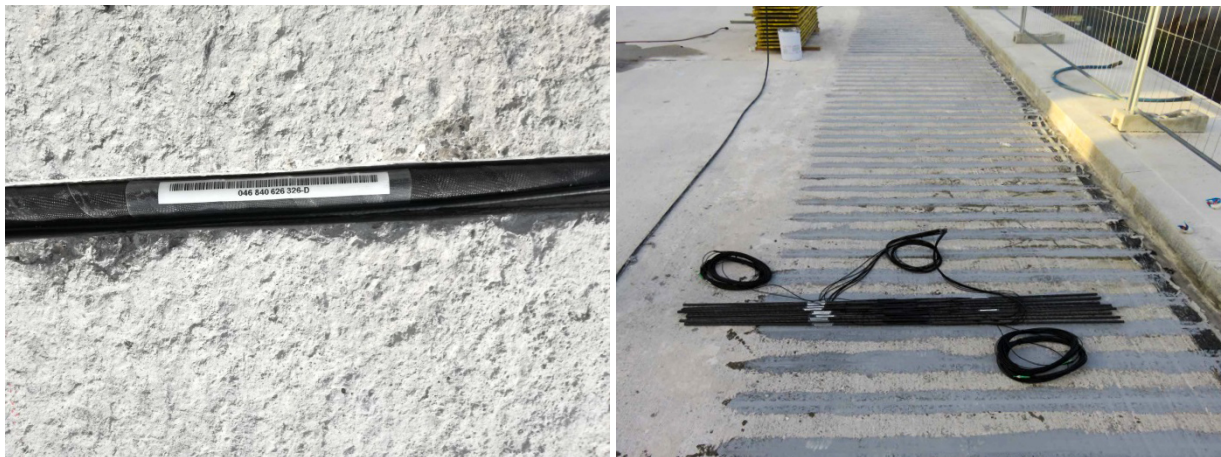
Figure 10: FBG sensor glued on carbon rod (left) and installed carbon fibre rebars on the right viaduct (right)
