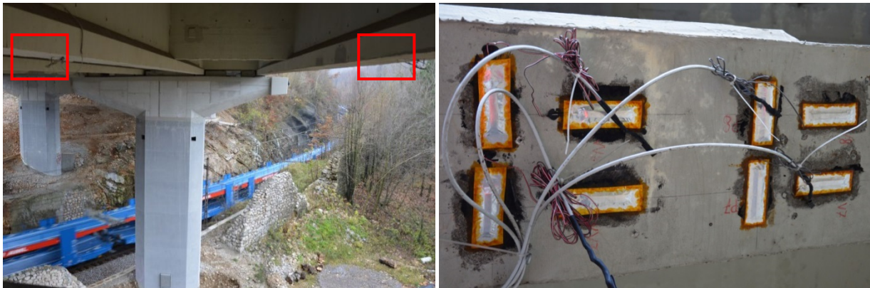
Figure 5: Two strain gauge locations on external and internal beams of the right viaduct – marked with red line (left) and 4 strain gauge sensors, all mounted at the same location on external beam of the left viaduct (right)
