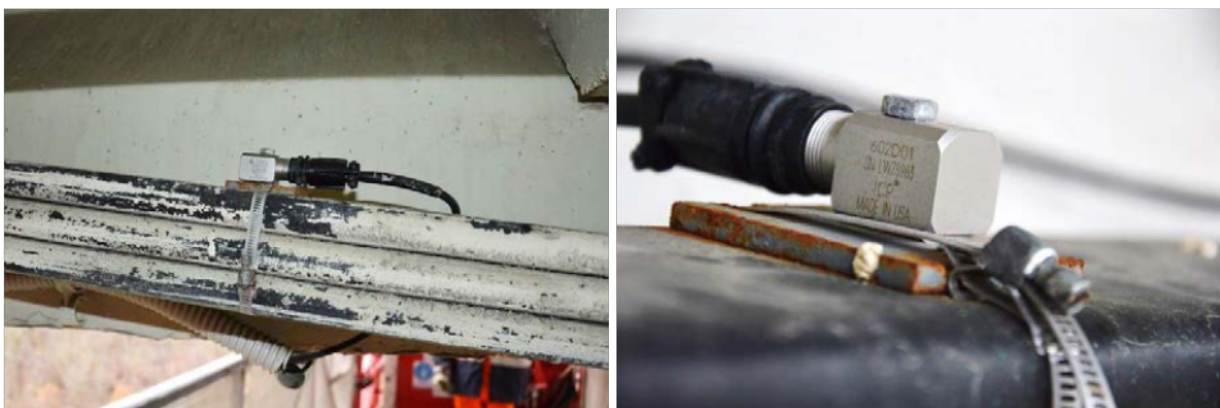
Figure 8: Prestressing cable consisting of 3 HDPE tubes and overall 6 strands with accelerometer (left) and accelerometer (right) on the left viaduct
