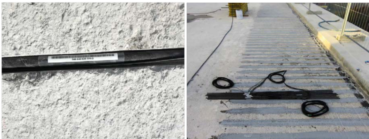
Figure 10: FBG sensor glued on carbon rod (left) and installed carbon fibre rebars on the right viaduct (right)
