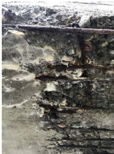
Figure 2. Corrosion process in down part of concrete slab
