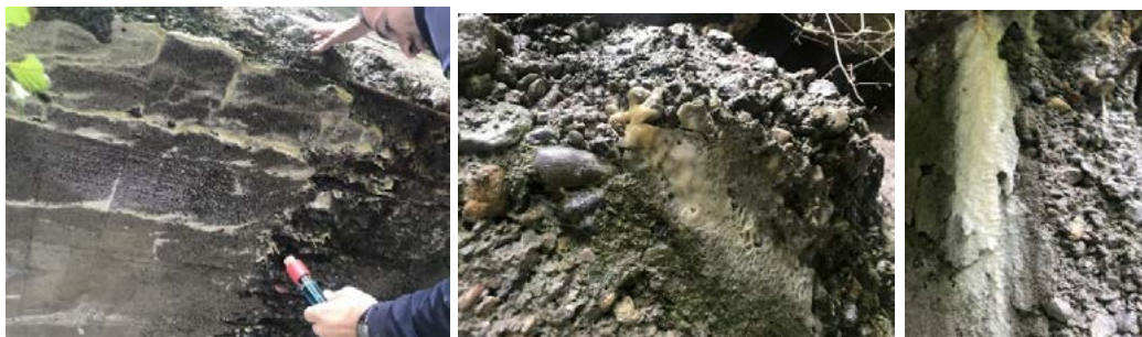
Figure 3: Degradation concrete elements
