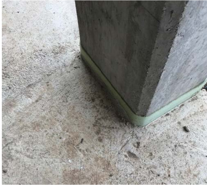
Fig. 13. No cracks around the column (age of 480 days). No special reinforcement around the column.
