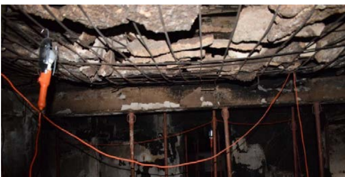
Figure 2: Spalling of concrete and collapse of RC slab defined
