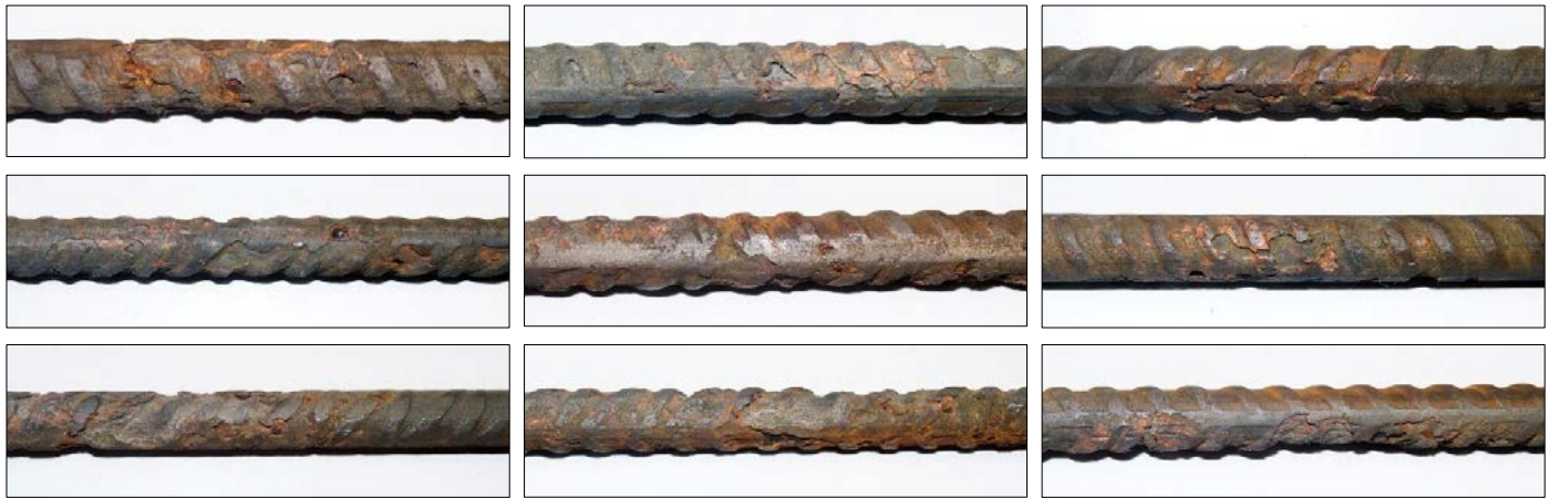
Figure 8: Localised corrosion (top: bar from specimen A2, middle: bar from specimen A3, bottom: bar from specimen A4)
