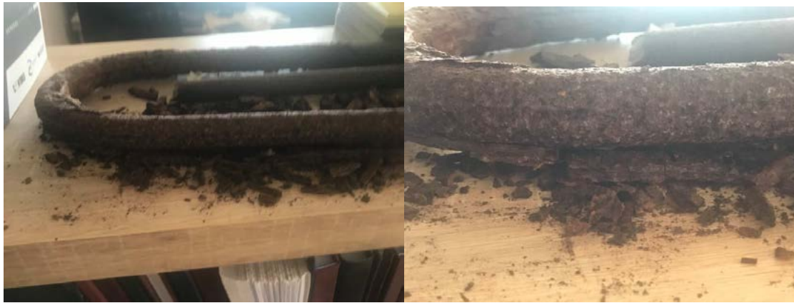
Figure 7. Reduction of armature cross-section caused by corrosion from direct contact with the external environment.
