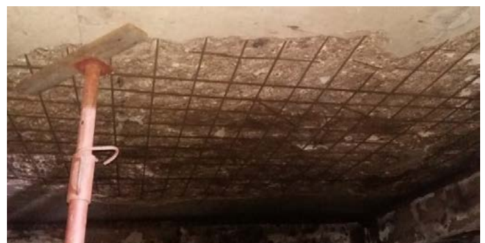
Figure 3: Falling off of concrete cover of RC slab defined with
