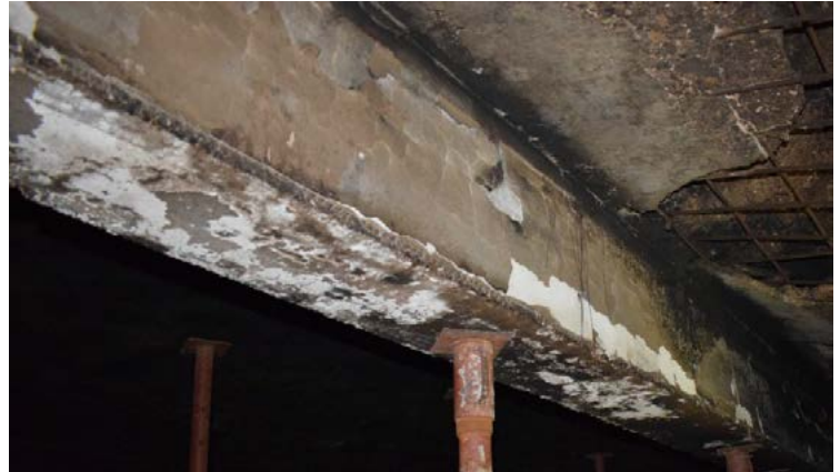
Figure 5: Micro and macro cracks in RC beam
