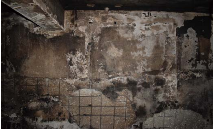
Figure 4: Falling off of concrete cover of RC wall
