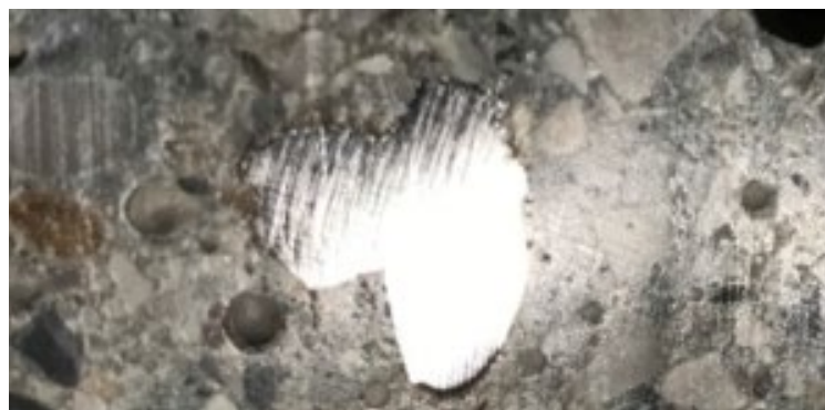
Fig 11. Steel rebar in a cylinder sample taken from the casted slab.
