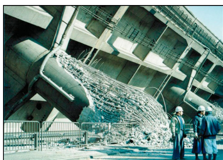
Fig. 2: An example of poor seismic design: the Hyogo-Ken Nanbu earthquake in Japan, 1995 42 (© Copyright 2018, Lecturas Digitales SA de CV)
