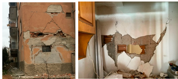
Figure 1. In-plane and out-of-plane infill walls damages (Elazig Earthquake, 2020).
