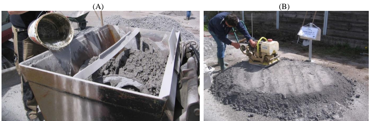
Fig. SI4 (A) Mixing of DPSA and DPS for preparation of D80/20 demonstration test field TP 1.2; (B) compaction of D70/30 (layer 2) on the TP 2.1 demonstration test field.
