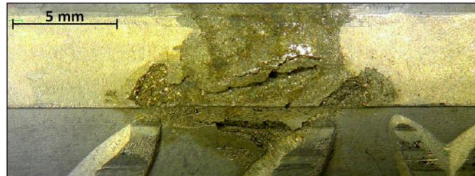
Figure 7. Optical image of the most severe corrosion damage found on a stainless steel reinforcement in concrete column C11 (located in the dry zone).
