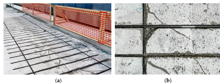
Figure 7. FBG sensors on the carbon fibre rods (span P13D): (a) Distance view; (b) Close-up view.
