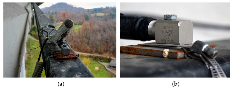
Figure 8. Accelerometers on the external prestressing tendons: (a) Distance view; (b) Close-up view.
