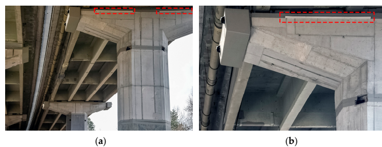
Figure 9. Long gauge deformation sensors (marked with red dashed line) on the pier: (a) Distance view; (b) Close up view.
