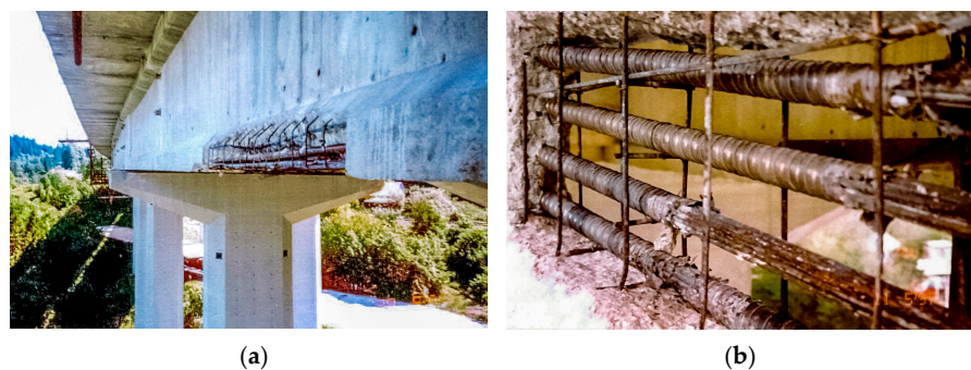
Figure 2. (a) Corroded prestressing tendons in I-shaped precast concrete girders of the viaduct deck; (b) Detailed view of the corroded prestressing tendons.
