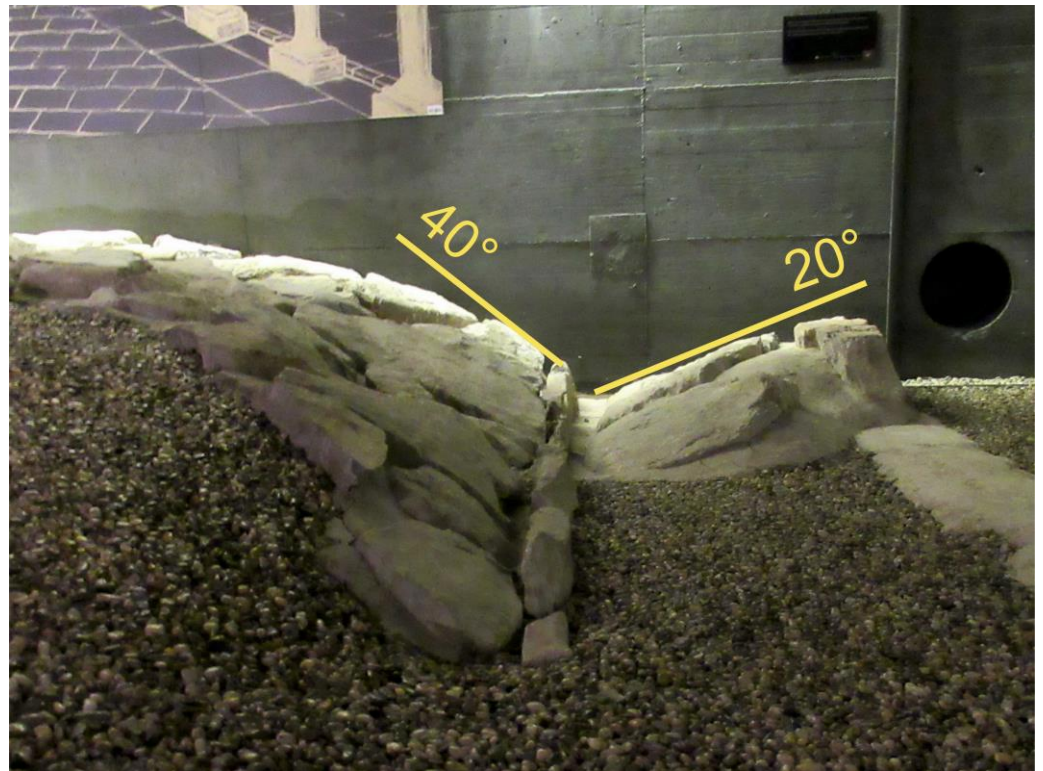
Figure 6. Deformed ditch paved with slabs along the southern edge of the road (location B on Figure 5). Road surface (left) is tilted by 40^\circ . The adjacent flagstone of the horizontal sidewalk is tilted by 20^\circ towards the road surface. Field of view is 1.8 m wide. View to east. Archaeoseismological Database (ADB) photo #4459. For location, see Figure 3.
