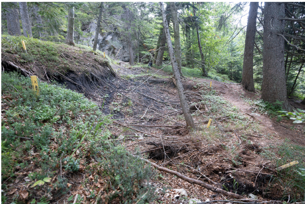
Fig. 10. Position of local road that crosses the Urbas landslide. Cross-sections represent the position of the road's left shoulder, which has been manually digitalised in orthophotos.
