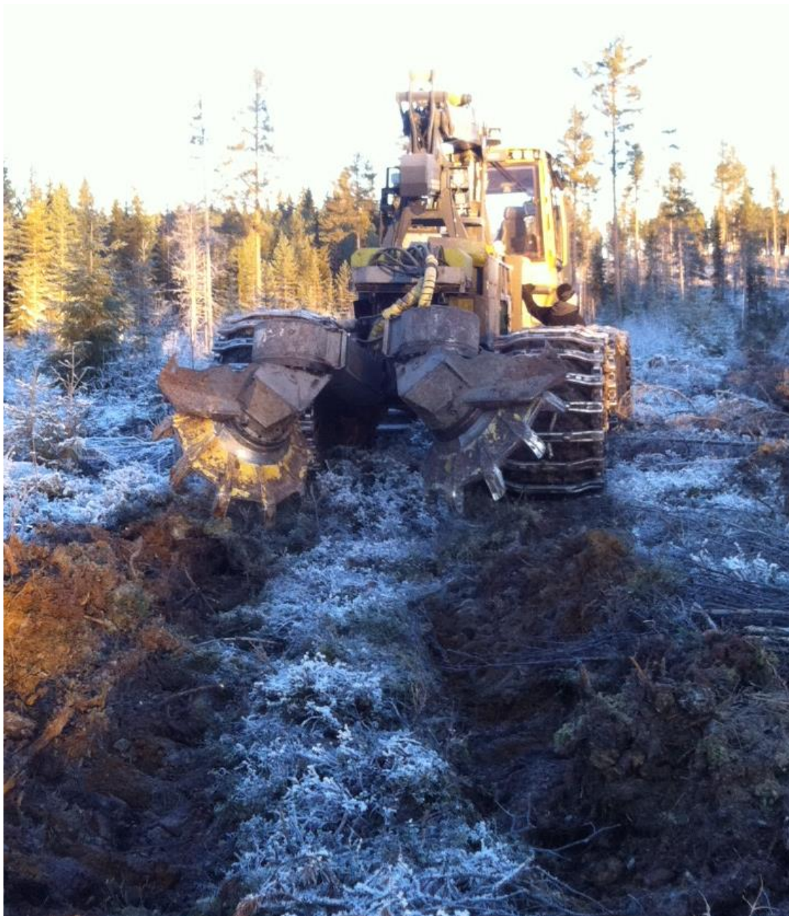
Figure 52: Mechanized site preparation using a Bracke T26 two-row disc trencher in northern Sweden in late November 2018. The trenching unit is mounted on a large forwarder, and the trenching can be performed as long as the soil is not significantly frozen (slight frost and snow is not a problem) (© Back Tomas Ersson, SLU).
