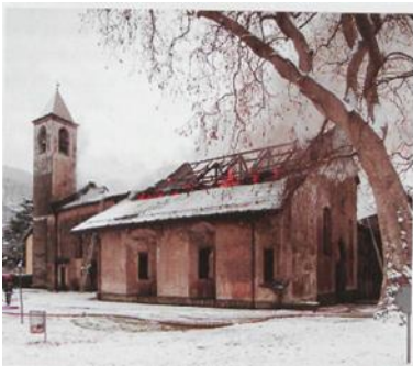
Figure 65 External view of the Church of Santa Maria delle Grazie after the fire occurred on the 31 December 1997. Photo by Fabrizio Savioli
